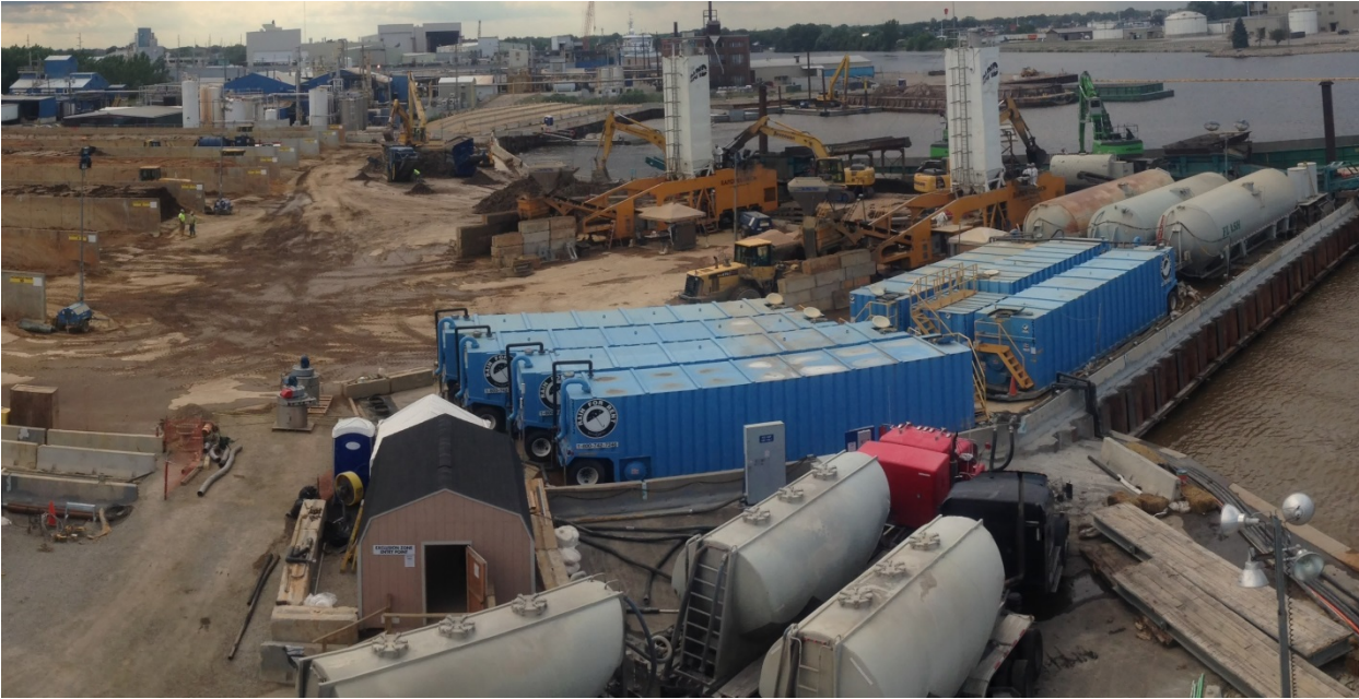
View of the Pugmill Mixers and Chemical Storage Tanks
